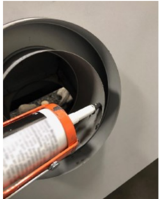
Figure 6.10 - Silicone Inner Exhaust on Fireplace
