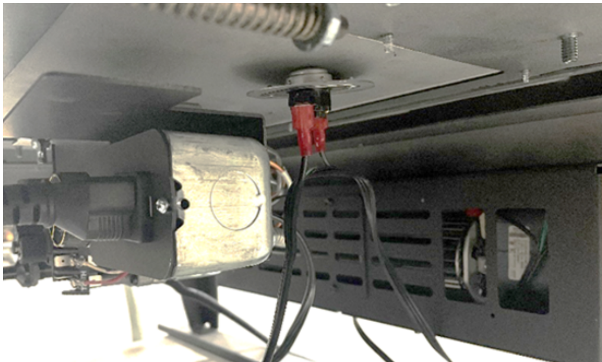
Figure 6.12 - Temperature Control Switch Location
